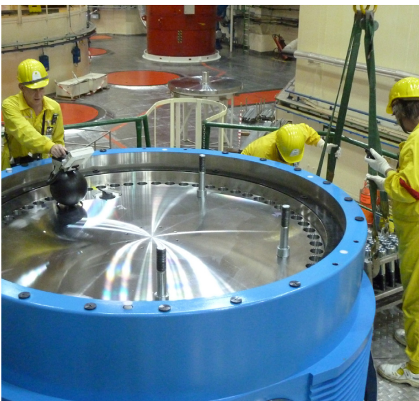
Dukovany NPP spent fuel cask closing ©CEZ
