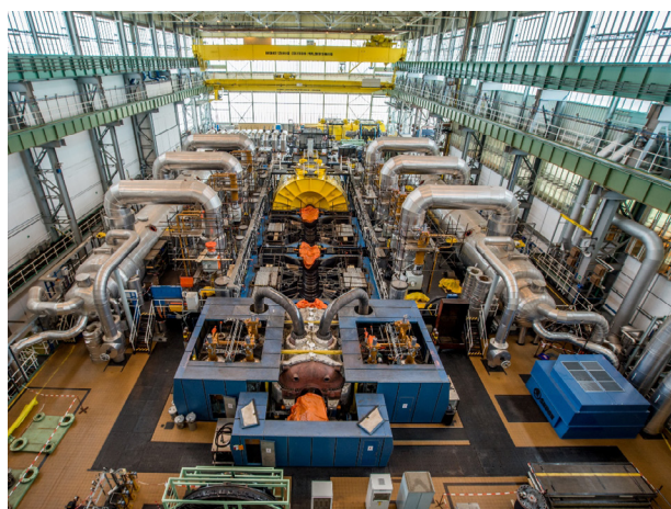
Temelin NPP turbine hall ©CEZ
